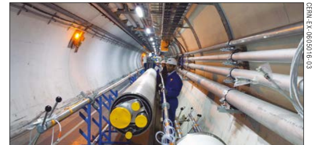
Fig. 3. Installation of the cryogenic distribution line (QRL) in LHC sector 1-2, the last to be equipped, in May 2006. Each sector involved placing 325 elements and carrying out almost 2000 internal welds.
