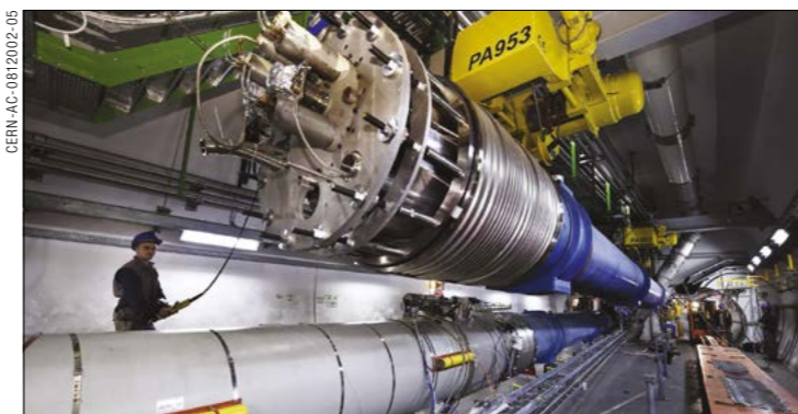
The transport of a 15 m-long, 35-tonne superconducting dipole magnet from LHC sector 3-4 to the surface in December 2008 in order to be repaired.
